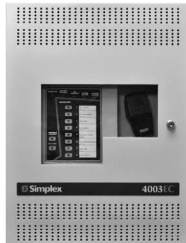
4003EC Voice Control Panel
