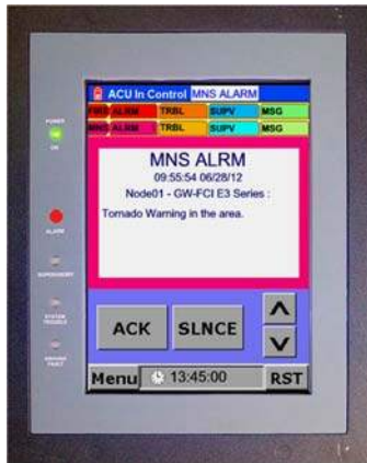
Figure 1 NGA Screen with MNS Alarm Event
